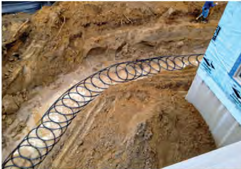
To reduce geothermal installation costs at Rivera Greens, Jens Ponikau of Buffalo GeoThermal Heating ruled out a vertical loop and a traditional horizontal loop, opting instead for a stacked slinky loop field. This system uses slinky coil rather than straight pipe, which is stacked in a horizontal trench, one at a depth of 8 ft. and a second directly above it at 5 ft.
