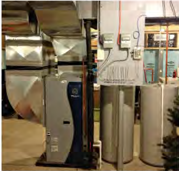
Sizing the geothermal equipment was a challenge for Buffalo GeoThermal Heating. High-performance WaterFurnace 3-ton 5 Series units were installed in order to meet the unique heating and cooling requirements of each homeowner at Rivera Greens.
